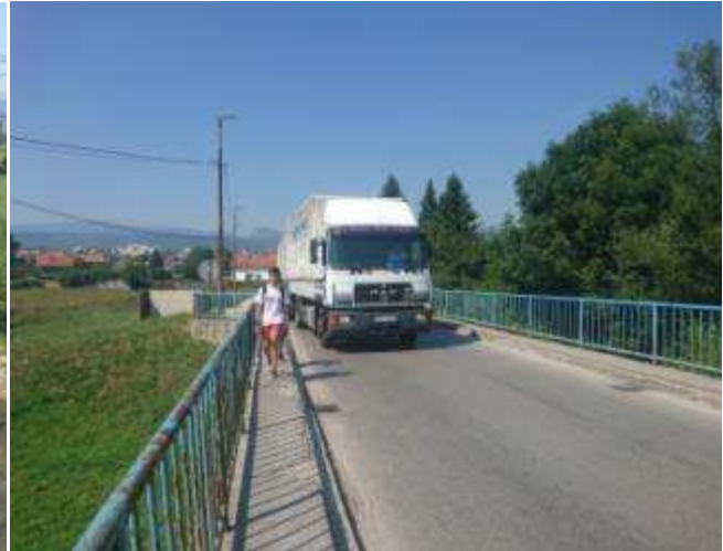
d) existing bridge, poor pedestrian safety conditions
