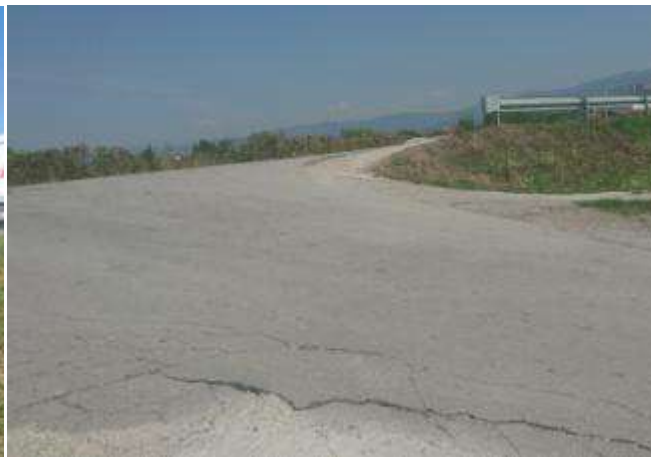
b) future connection point of the temporary route across the river and the existing main road
