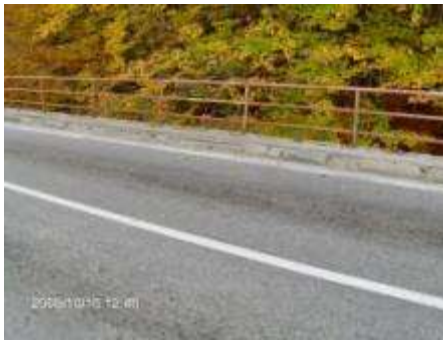
e) Damaged pavement structure, turning point
