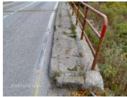
f) Damaged fence
