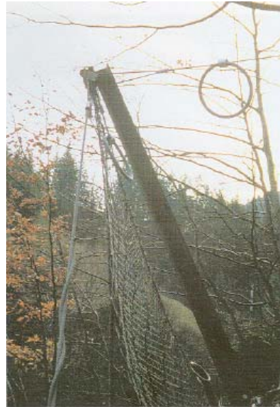
Slika 6.47: Protection of Hrušica Vrba motorway against snow avalanches and rock falls by rockfall protection nets made of steel weaving
