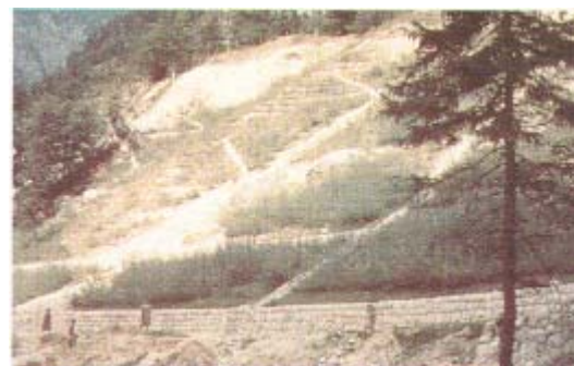
Figure 6.44: Arrangement of surface and deep drainage and biotechnical stabilisation of the slope
