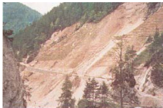
Figure 6.42: Rehabilitation of slope - slide by wattles, live stakes, grass planting and afforestation
